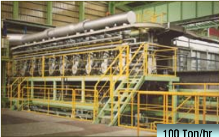
60 Ton/hr Pusher type 3-zone continuous reheating furnace
